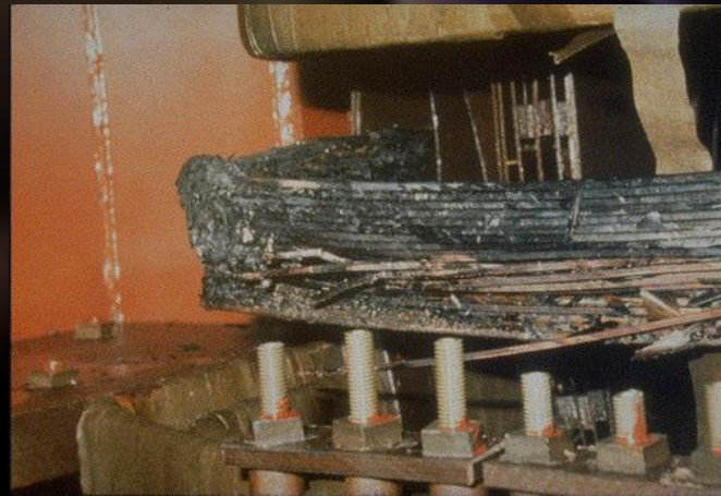
Transformer damage in New Jersey after March 1989 geomagnetic storm. Credit: Public Service Electric and Gas and Peter Balma
